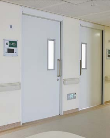
Doors for wards
